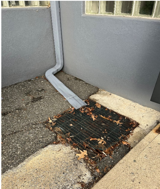
Figure 20: Outdated and ineffective stormwater management facilities.
