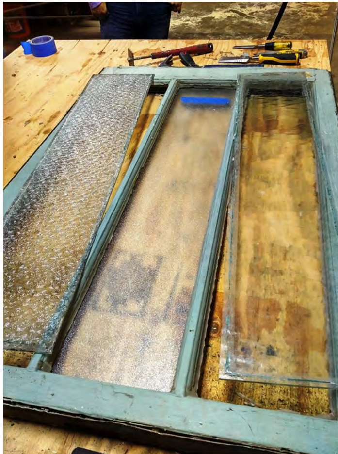
Typical condition of lavatory hopper windows in 2016.
