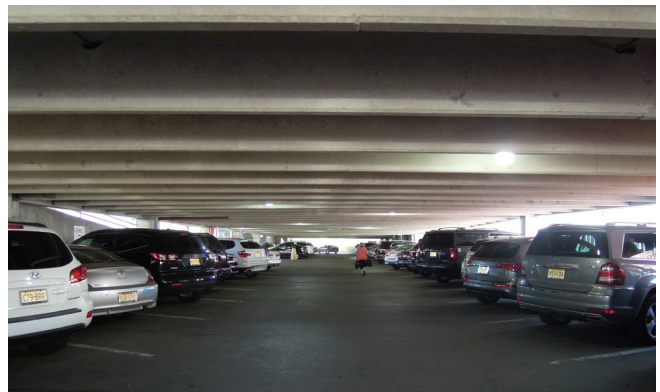
B.8-03: Minimal floor to floor heights within the North Fullerton Deck create dim spaces that don’t feel safe.
