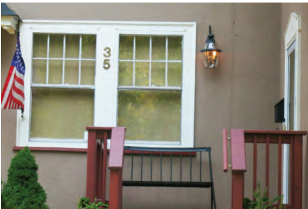
Stucco is available with integral colors, but if light power washing and cleaning solutions do not remove stains it can be painted in any shade using compatible primers and finish layers.
