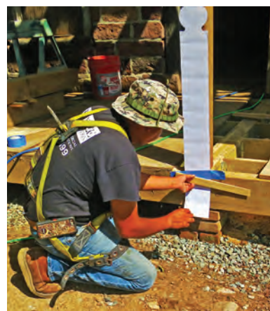
Many projects on historic buildings include a range of actions from maintenance through replacement. Left: templating a replacement newel post for a porch.
