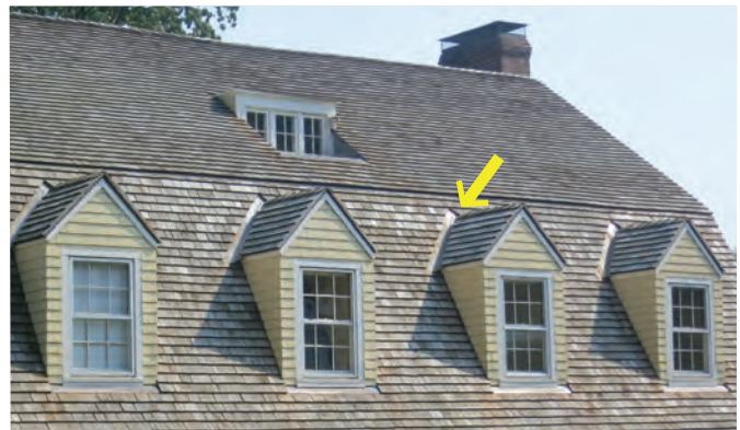
Wood shingles can be treated to provide resistance to fire or decay. Flashing (arrow) at dormer valleys and all intersections is key to a roof’s longevity.
