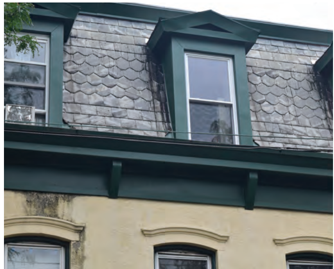
Luckily, many important buildings retain original materials that lend pleasing character and texture to the streetscape. When maintained, natural materials like the decorative slate shown here last a century or more.
