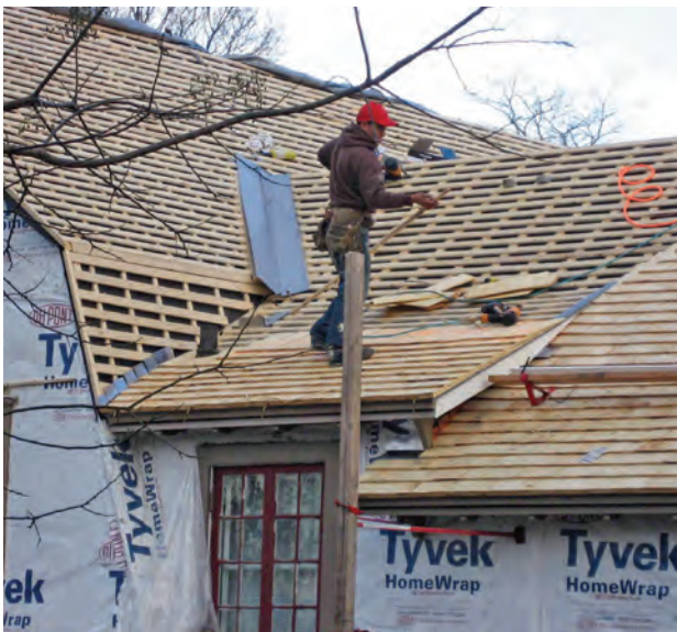
Left: Additional roof furring or equivalent spacer systems provide ventilation for the shingles above, over a protected sub-layer. Ventilation under cladding to promote drying enhances the longevity of insulated walls and roofs, which used to be dried by waste heat through uninsulated walls.
