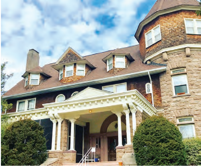
Note the rounded entry arch and the circular stone and shingle corner tower, identifiers of the Richardsonian Romanesque style.
